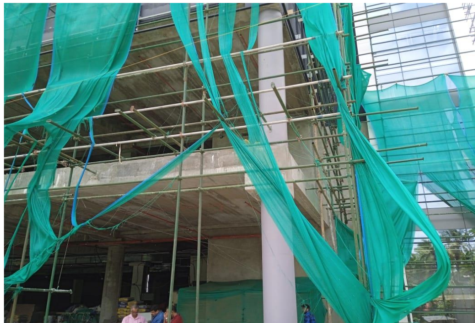
Figure 5.4 M/s Kalyan Silks building, Thodayad Junction, Kozhikode. Failure to provide quality safety net to prevent accidents. Photo taken by Audit party on 20 September 2023.
