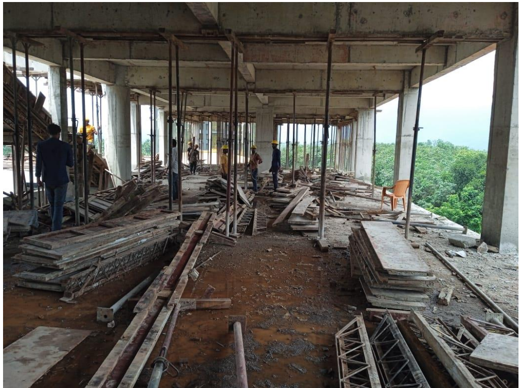
Figure 5.5: M/s Hillsinai building, Markaz Knowledge City, Kaithappoyil, Kozhikode. Work ongoing in the site even after issuance of stop memo. Photo taken by Audit party on 21 September 2023.
