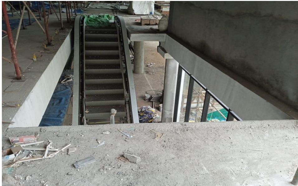
Figure 5.3 M/s Kalyan Silks building, Thodayad Junction, Kozhikode. Failure to cover or guard suitably and properly every open side, into or through which a building worker, vehicle or lifting appliance may fall. Photo taken by Audit party on 20 September 2023.
