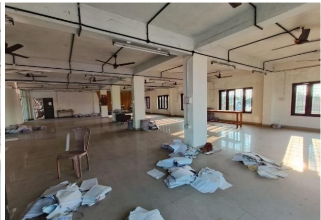
Figure 5.2: Floor 3 of BOCWWB Ernakulam District Office building, Edappally not rented out and lying vacant. Photo taken by Audit Party on 11 October 2023
