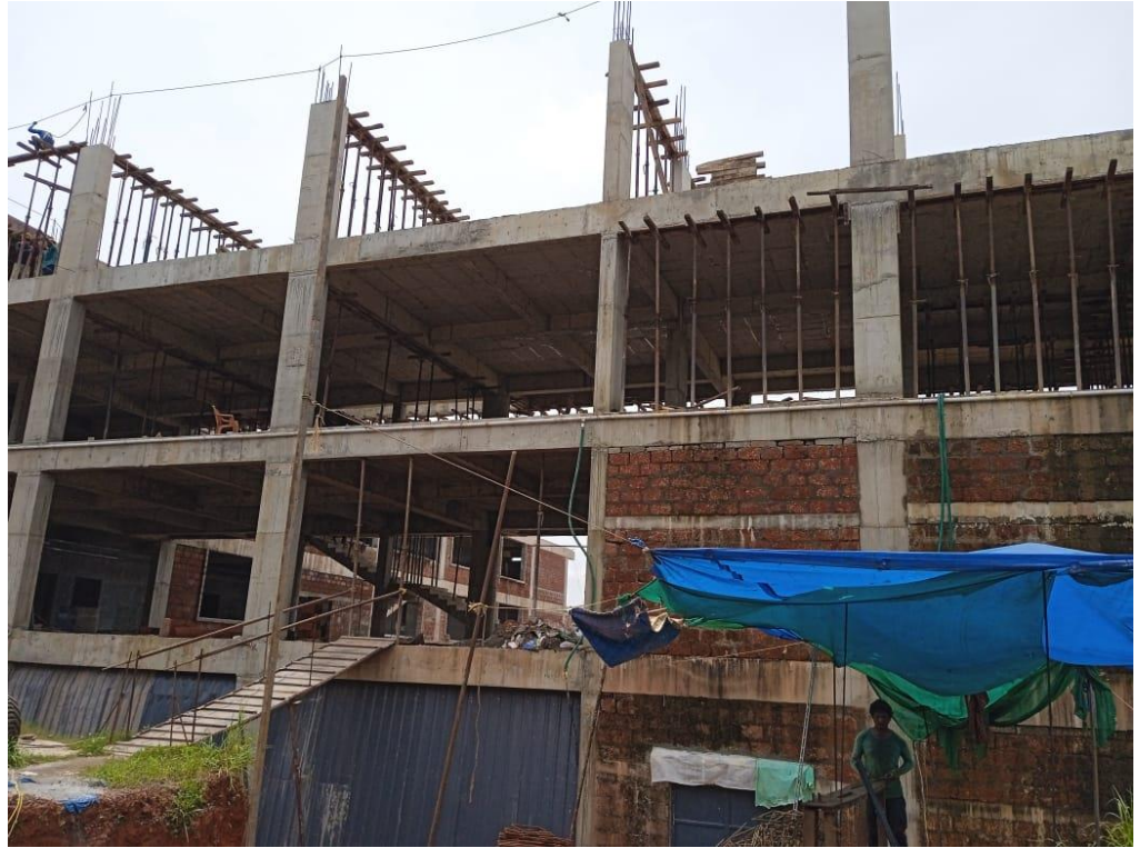
Figure 5.6: M/s Hillsinai building, Markaz Knowledge City, Kaithappoyil, Kozhikode. Failure to provide safety net of standard. Photo taken by Audit party on 21 September 2023.
