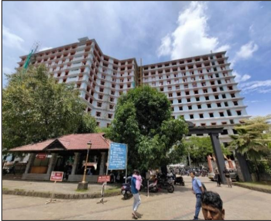
Figure 5.6: Unauthorised construction at Amrita Institute of Medical Sciences, Kochi Corporation
