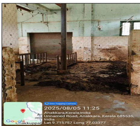
Figure 3.3: Cow dung dumped inside the slaughterhouse at Chakkupallom
