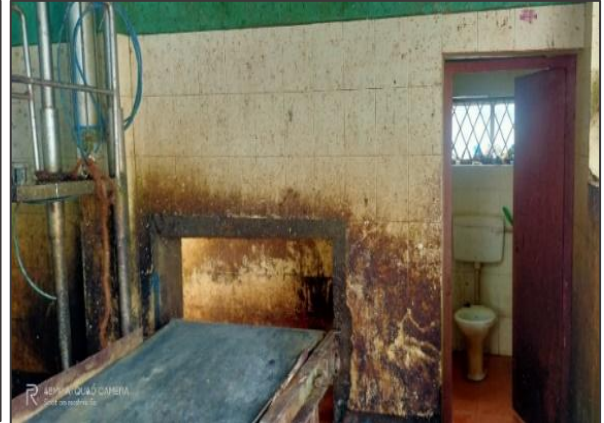
Figure 7.2: Dirty walls and unusable conveyor belt
